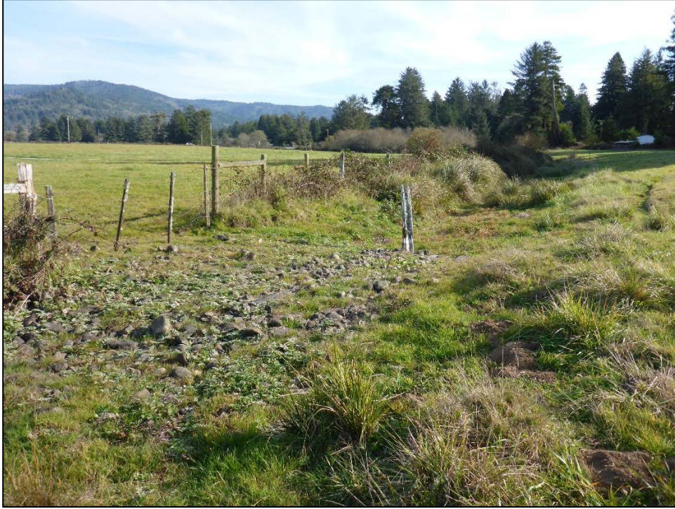
Figure 2-6. Low-water crossing with buried culverts overlain by placed cobbles, located in the middle of Reach 2 (looking downstream). (November 2019).
