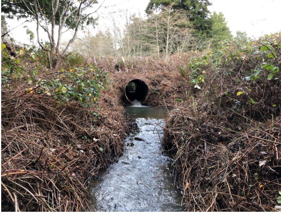
Figure 2-13. Middle Stotenburg Creek crossing at Fred Haight Dr. Culvert is 5 feet in diameter.
