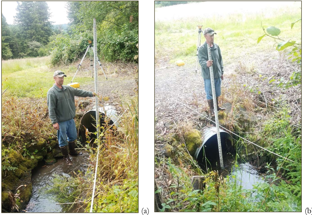
Figure 3-2: Existing CMP stream crossing set at a reverse grade with RSP along both banks, (a) outlet slightly embedded and poorly aligned, and (b) poor inlet alignment and aggradation upstream of culvert. Photo courtesy of SRA.
